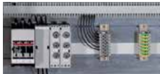
Mains distribution board
